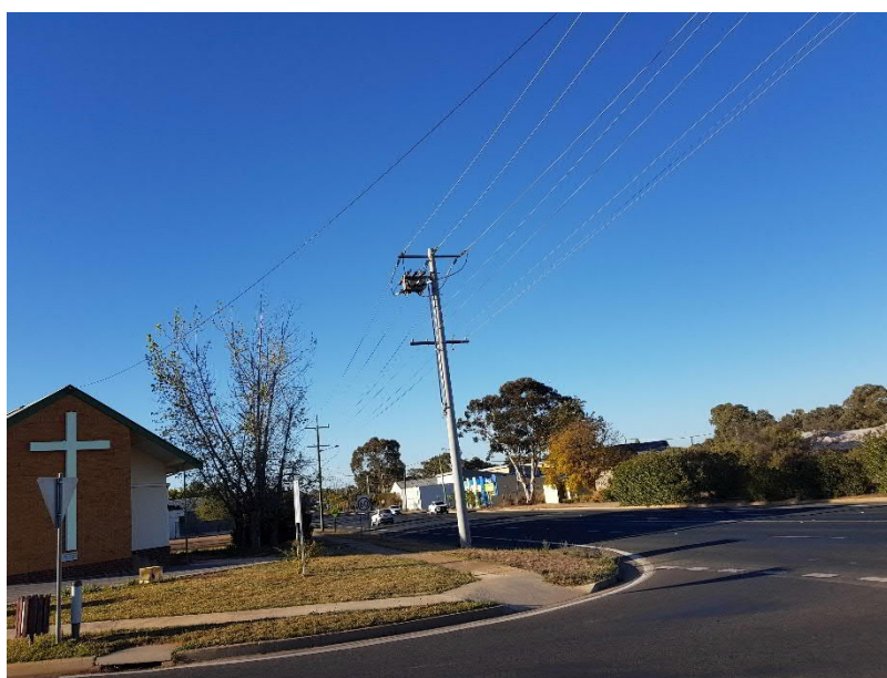
Photo 5 – Existing transformer on Silver City Highway (facing south from southwest corner of site)
