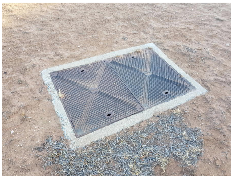
Photo 7 – Existing Telstra pit on Pitman Avenue
